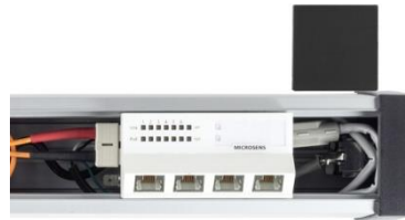
Micro Switch installed with a downlink in an MS140131GT-8
