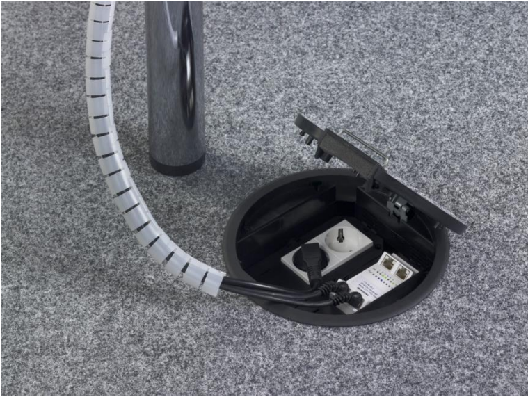
Underfloor system open
