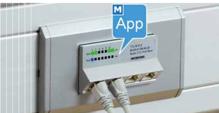
MICROSENS Micro Switch mounted in a cable duct
